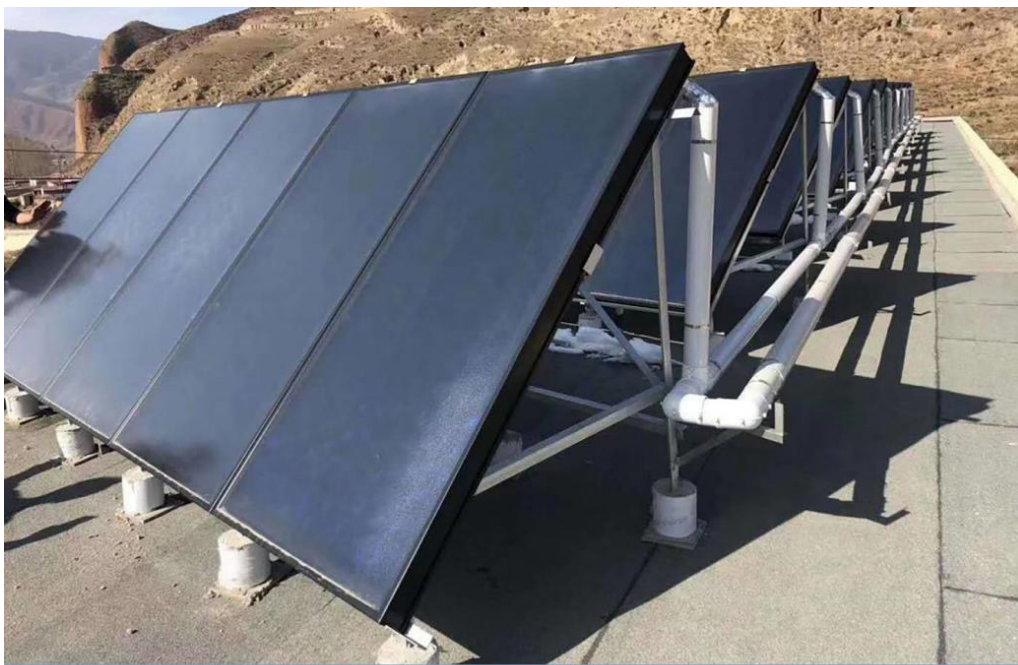
Concentrated hot water supply system, France, 2021
